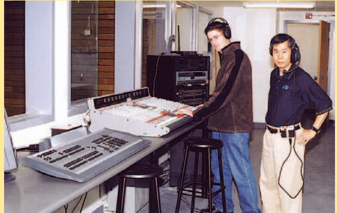
Inland AV personnel commissioning the audio and stage lighting systems in the Performing Arts Centre in Dryden, Ontario.
